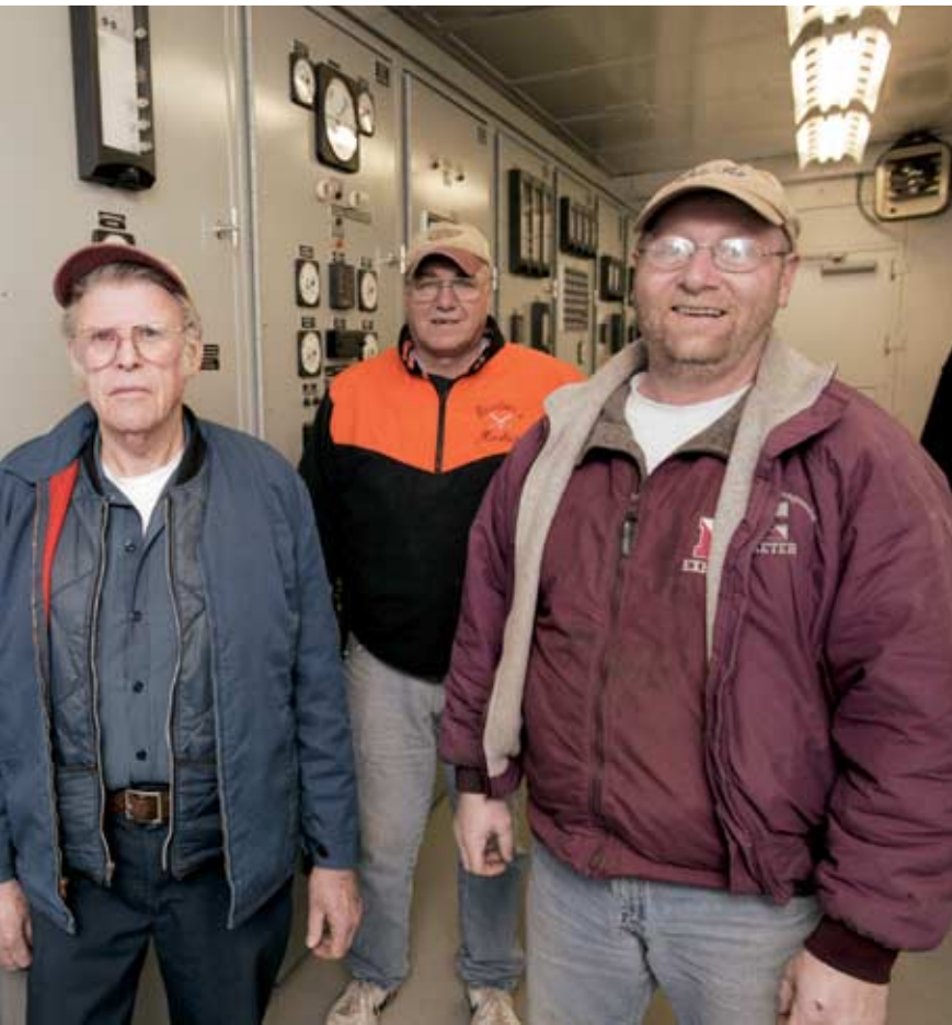
Helping the Academy conserve energy is a new high-voltage yard, which enables facilities management to better control energy distribution on campus. Responsible for overseeing the yard are electricians (left to right) Ralph Moreland, Joe Keraghan, Bob Boyd and electrical shop supervisor Dennis Bolduc (not shown).
